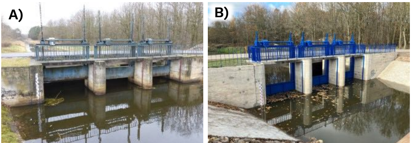
Figure 8: Before (A) and after (B) renovation of the weir at Zamość, Kampinos National Park (PL). This restoration helped re-wetting 198ha of peatland.
